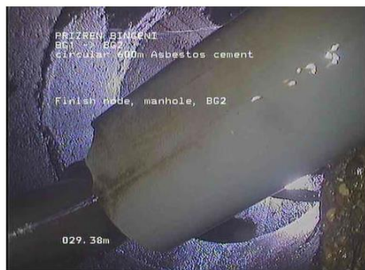
BG1 - BG2_0fd34358-8907-4c02-b518-b385a4a8d2e3_20230413_1 03129_583.jpg, 00:06:03, 29.38 m Finish node, manhole, BG2
