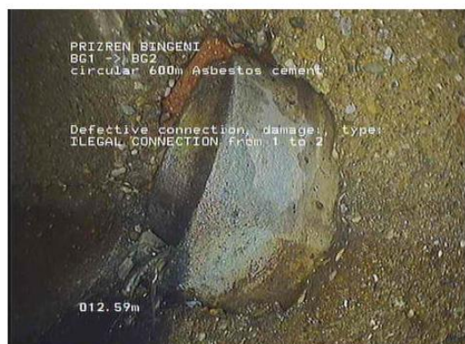
BG1 - BG2_ccf297cd-9415-417c-a245-393017405517_20230413_1 02444_511.jpg, 00:01:26, 12.59 m Defective connection, damage: type: ILEGAL CONNECTION from 1 to 2
