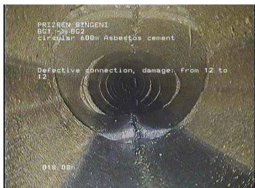
BG1 - BG2_b857c71d-0714-4041-9a6b-ddb811e57f83_20230413_1 02525_594.jpg, 00:02:05, 18.08 m Defective connection, damage: from 12 to 12
