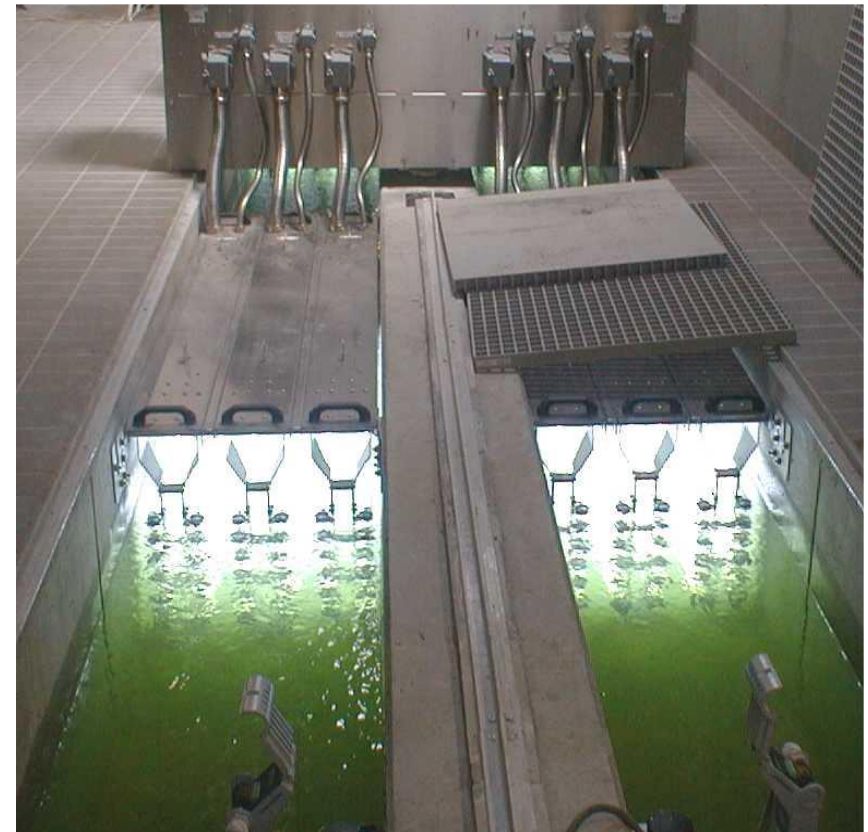
WWTP Bad Tölz: UV-radiation
